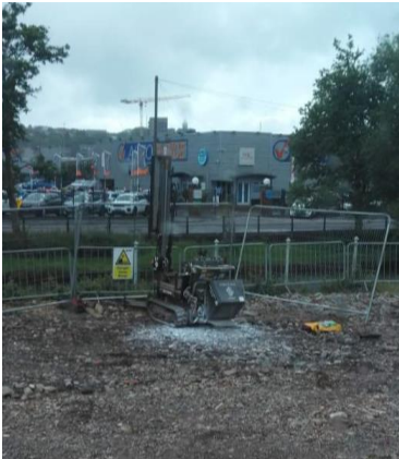
Figure 1: The rig after the incident
